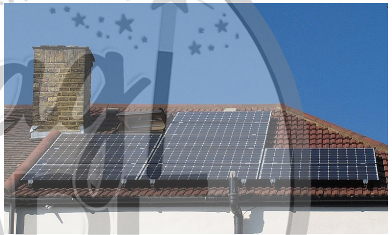
Solar panels on the roof of a home.
